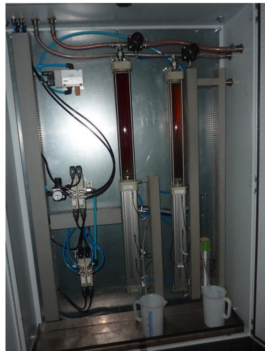
Pic. 2: Binder dosing cabinet with two piston pumps.
